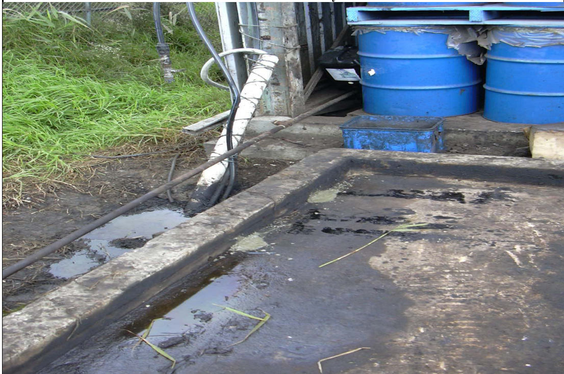
Plate 6 - Leakage of Wastewater to Land / Stormwater
